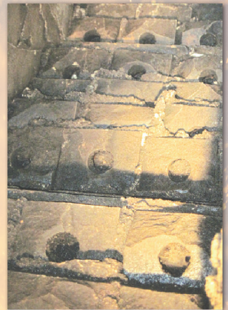
Jagged corbeling and exposed brick cores (holes) in smoke chamber
